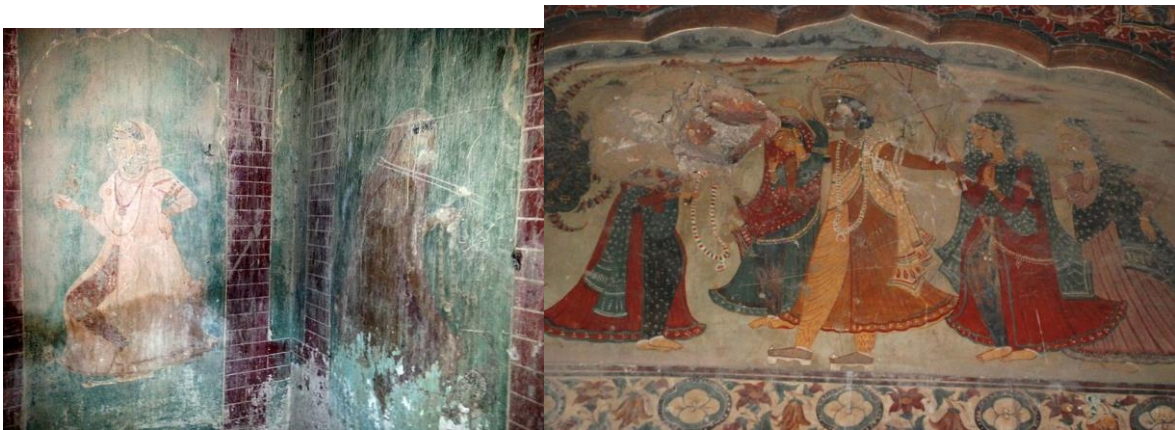
Present condition of wall Murals
