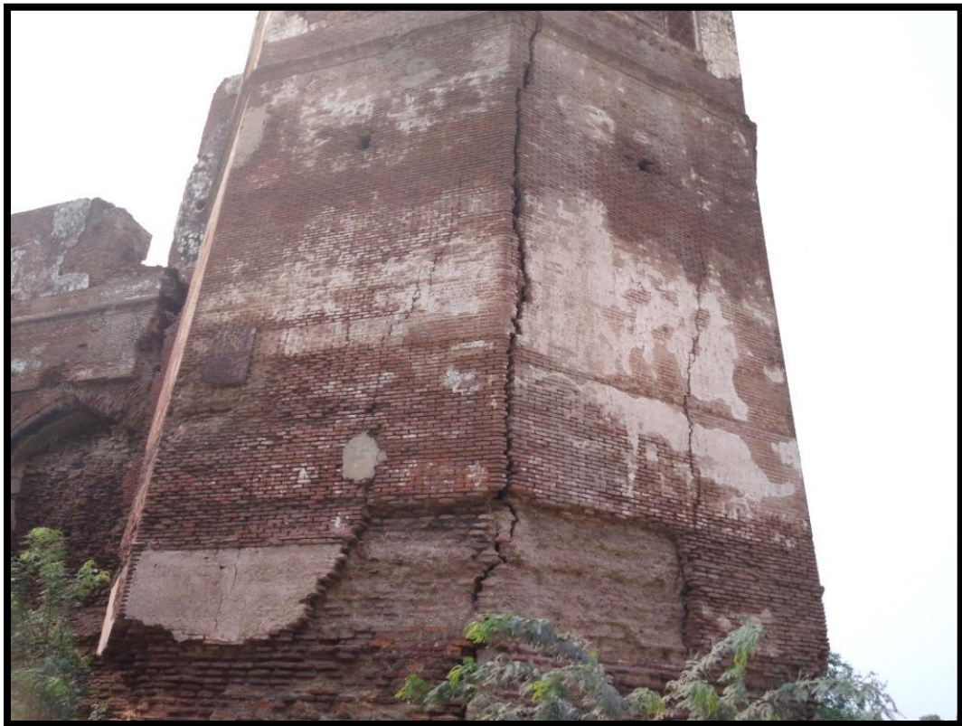
Figure 3 Cracks in Fort Wall Bannock
