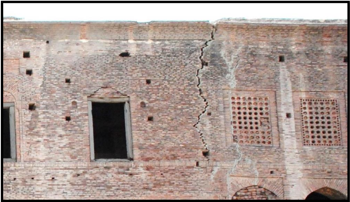
Development of Cracks in Sikh Haveli
