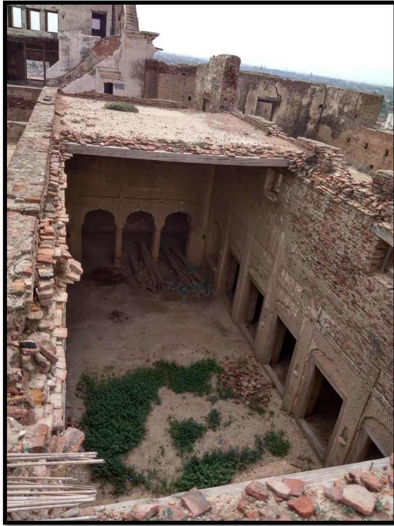
Present condition of Sikh Haveli
